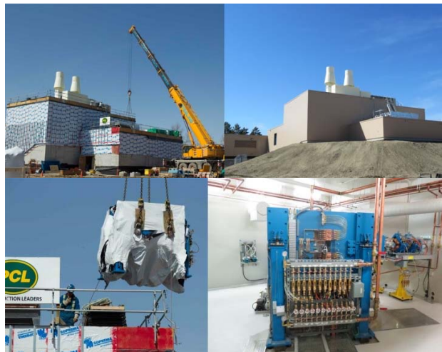
The Saskatchewan Centre for Cyclotron Sciences building (top row) in April 2014 and April 2015. The cyclotron (bottom row) being lowered into place, April 22, 2014 (left) and ready for use, December 2014.
